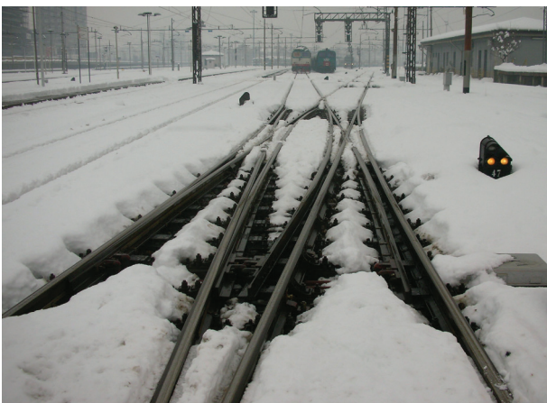
Typical Heated Points Systems - Milan, Italy.
